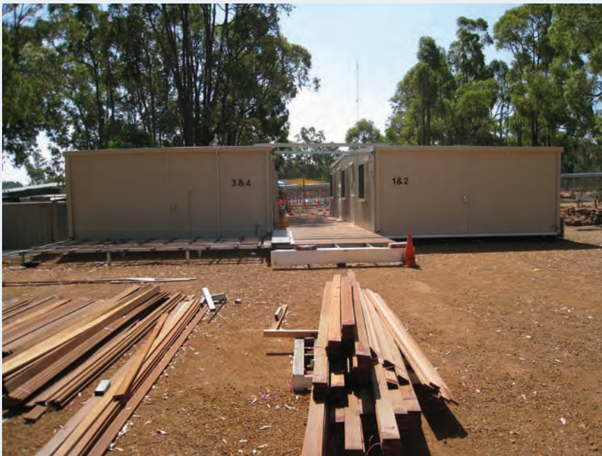
Two transportable units to be used as program rooms were being installed at the time of the inspection.
