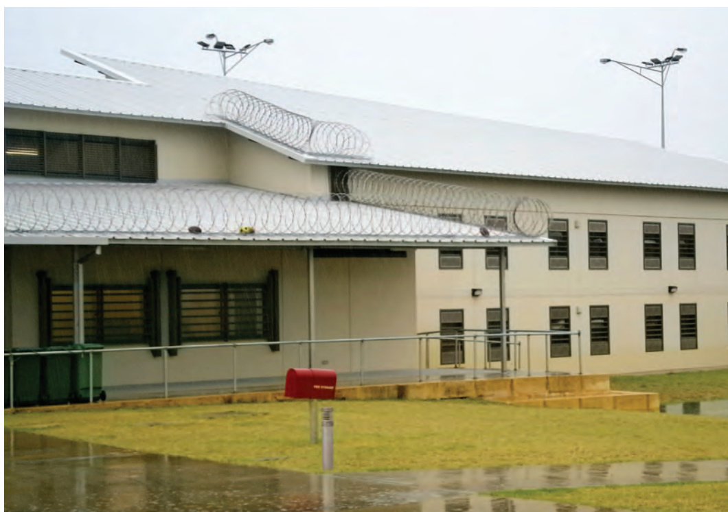
Photo 22: Razor wire retrofitted to roof edges to prevent ascents.
