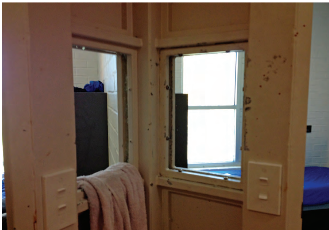
Photo 6: Example of cells breached via observation panels.
