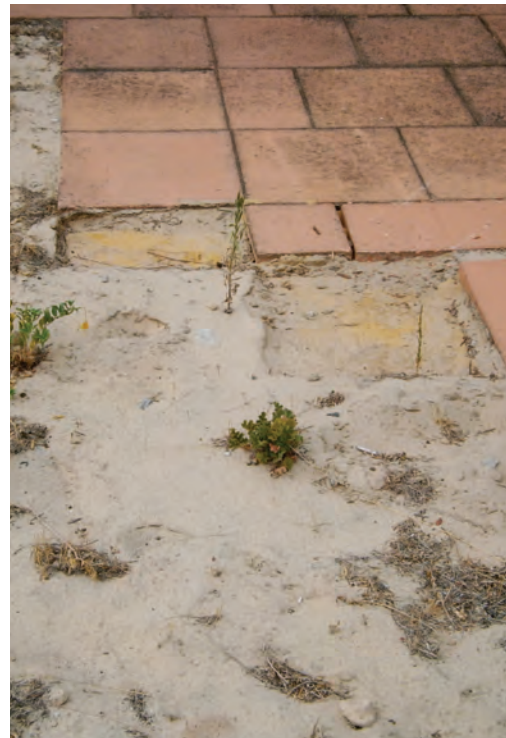
Photo 10: Unfixed pavers were easily accessed by detainees to use as tools.
