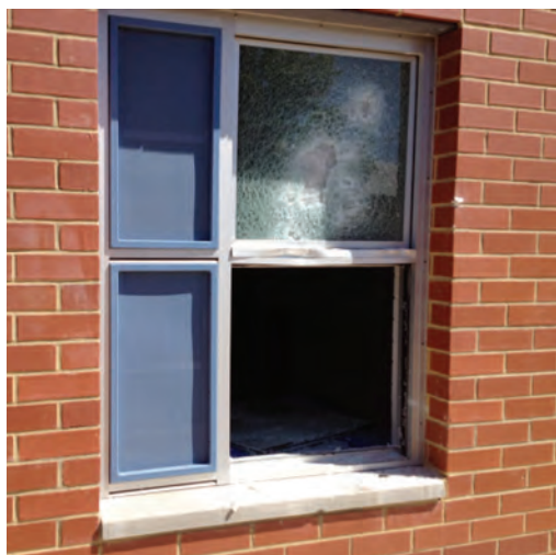
Photo 11: A Harding Unit window breached after external attack.
