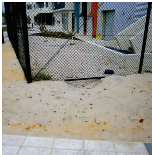
Photo 15: Detainees were able to tunnel under the fence due to soft sand and the absence of a concrete plinth.
