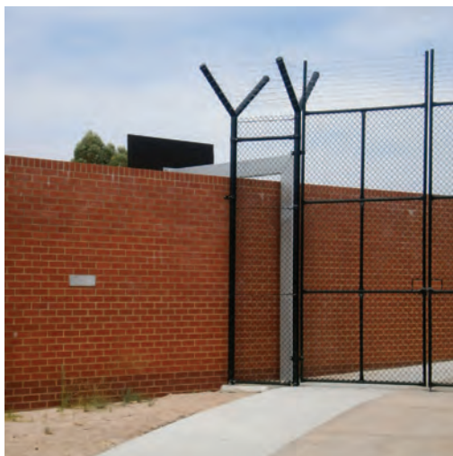
Photo 14: Lack of height continuity in management fencing. Detainees were able to easily climb the wire fence and access the lower brick wall, bypassing the barbed wire.
