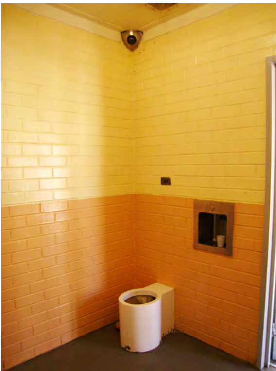
Figure 7: Toilet, water outlet & surveillance camera in a multipurpose cell.
