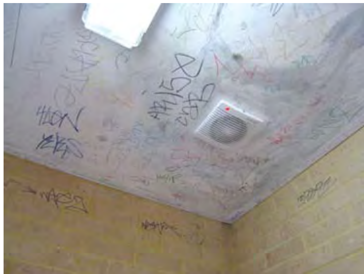
The ceiling of a toilet cubicle in the 'ed voc' area.
