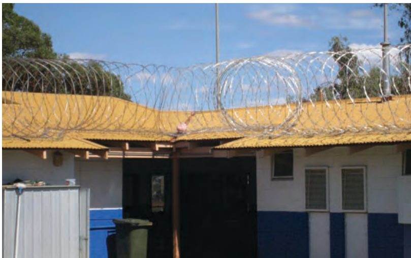
Razor wire on Unit 2 Minimum Security Roof [Note how easy access to the wire is. Note basketball on the roof and garden shed making access even easier].
