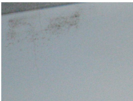
Mould on wall and ceiling of Medical Centre.
