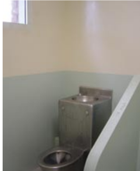
5. New toilet and drinking fountain unit installed in the South Hedland cells.
