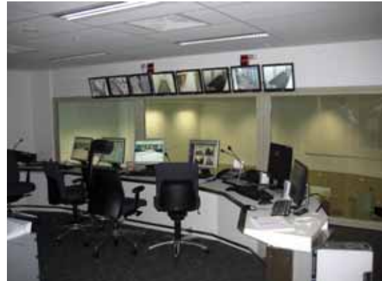
primary control room
