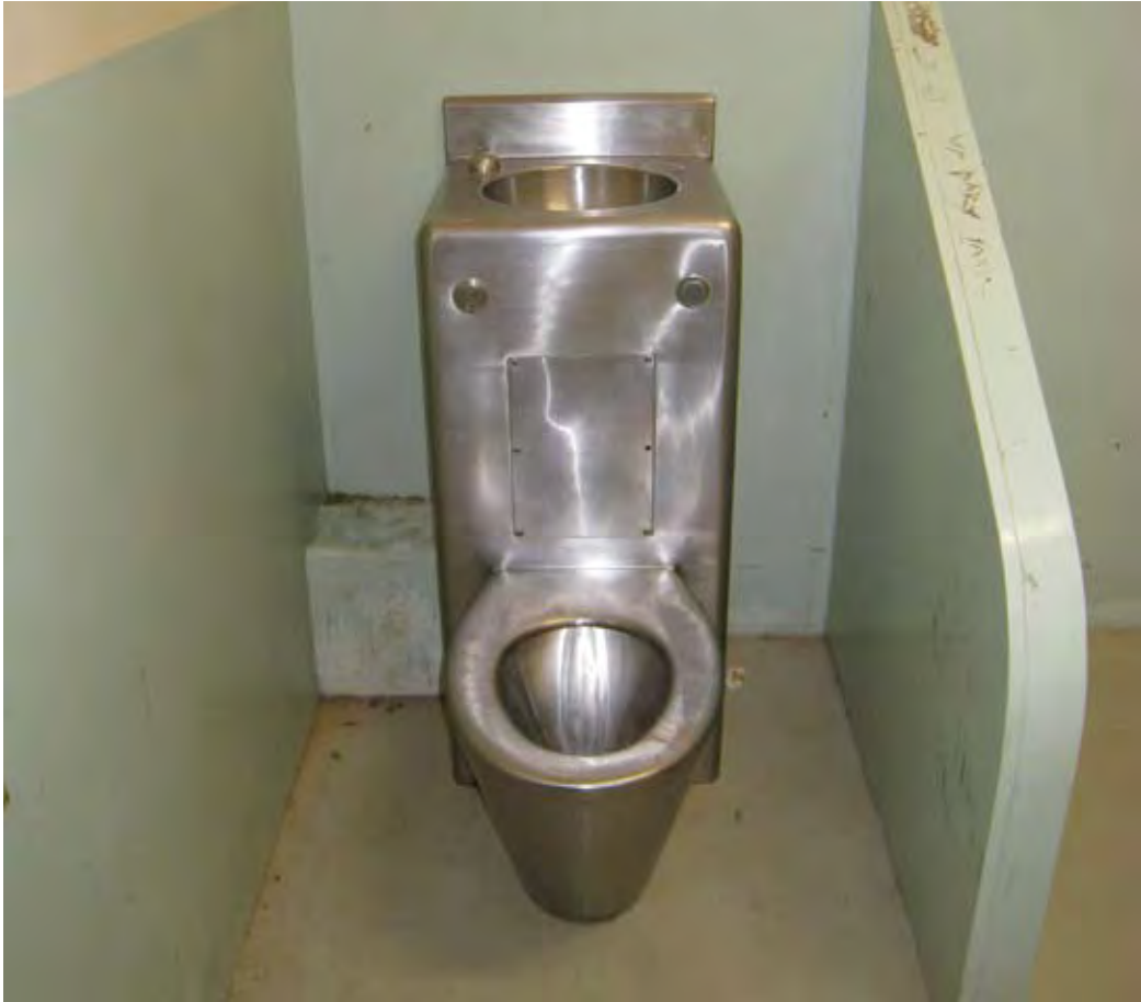
A rather filthy toilet installation in the holding cells at the South Hedland Courthouse. Persons in custody strongly object to having to use water fountains in such installations.
