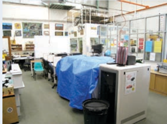
Tarpaulin laid over computer equipment as the Education Centre's roof leaks
