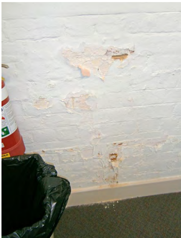
Photo 7: Result of rising damp at the Supreme Court custody centre
