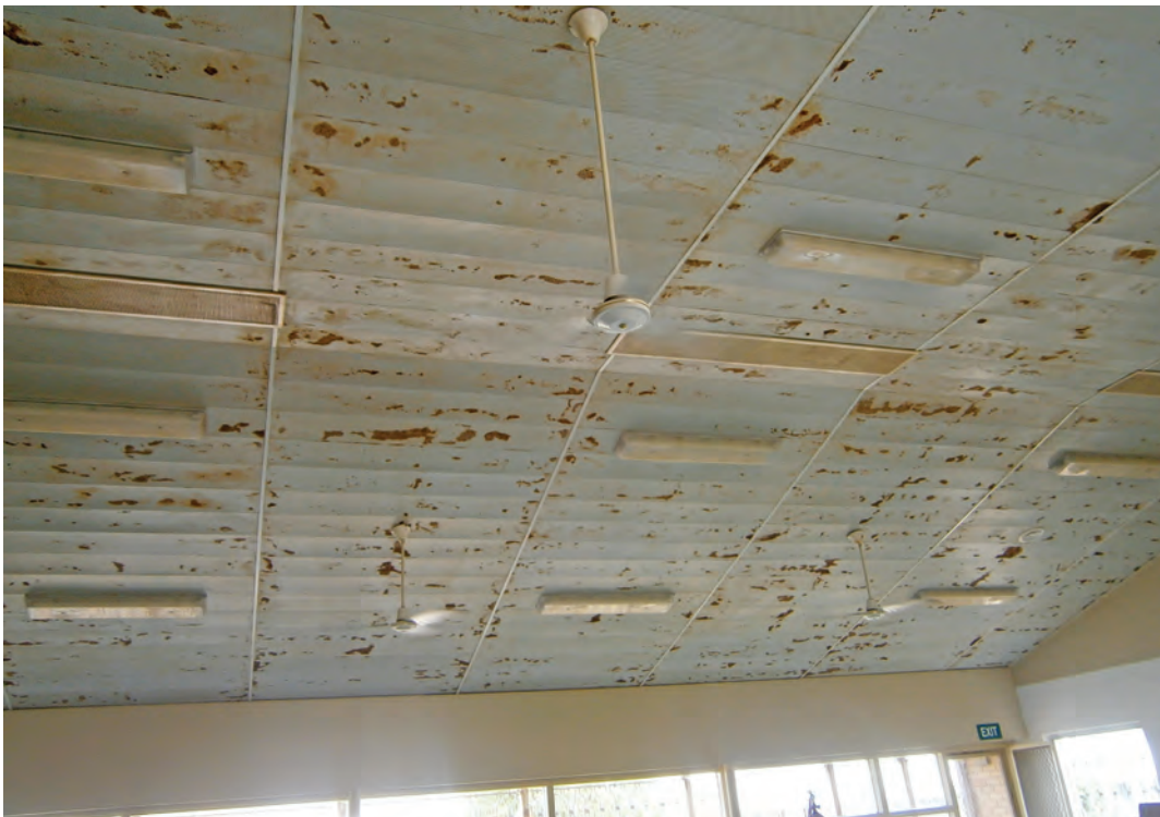
Photo 3 : The poor condition of the ceiling in Unit 2
