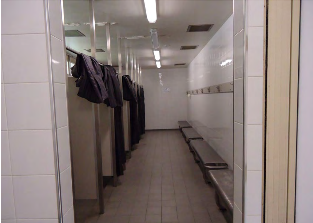
Figure 8: The newly refurbished bathrooms in Units 2 and 3 were of a high standard.
