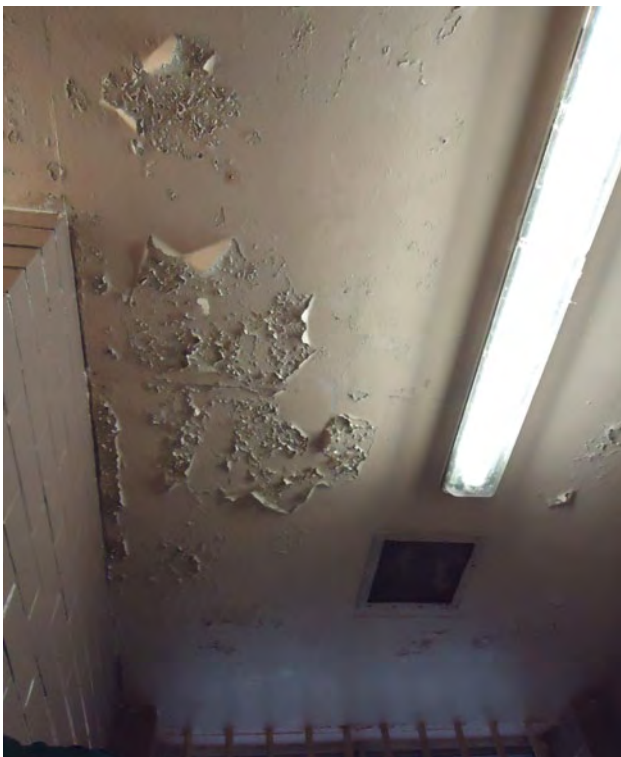
Figure 9: In contrast, the bathroom facilities in Unit 1 were in poor condition.
