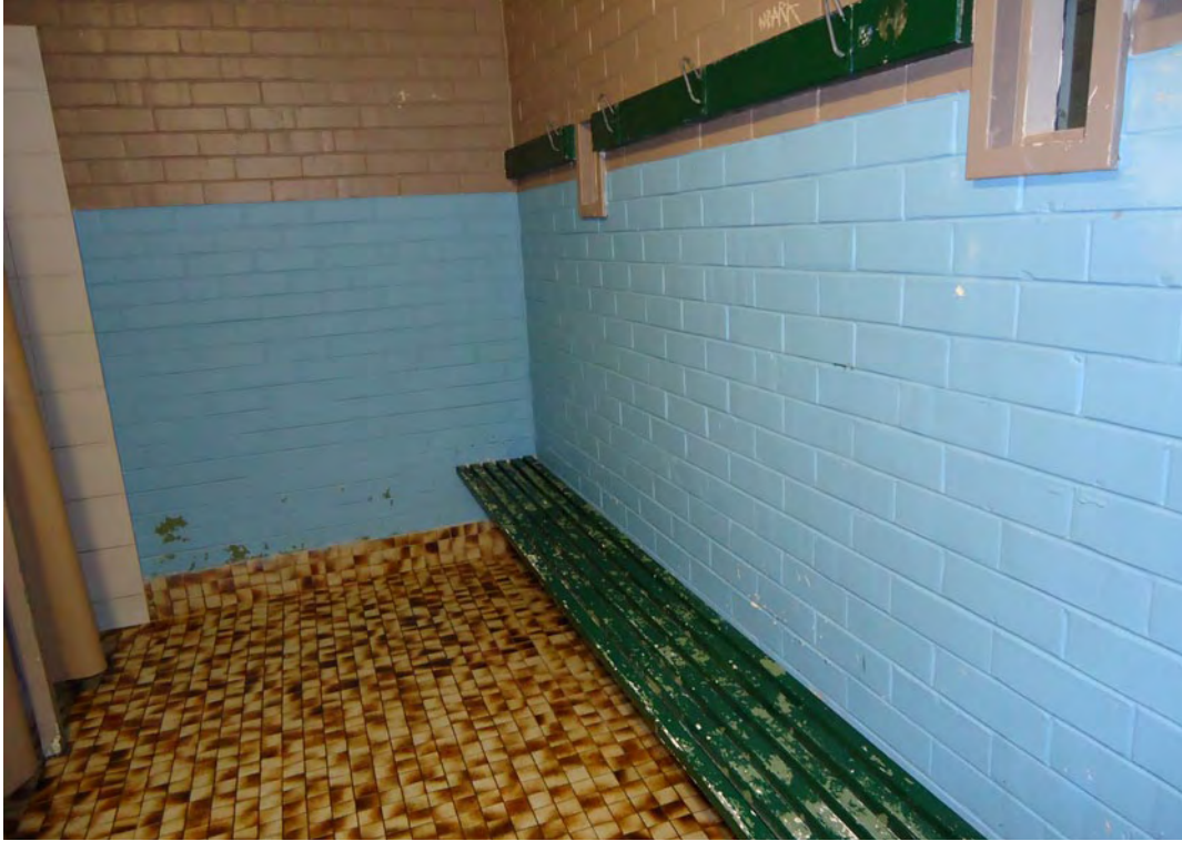
Figure 10: In contrast, the bathroom facilities in Unit 1 were in poor condition.
