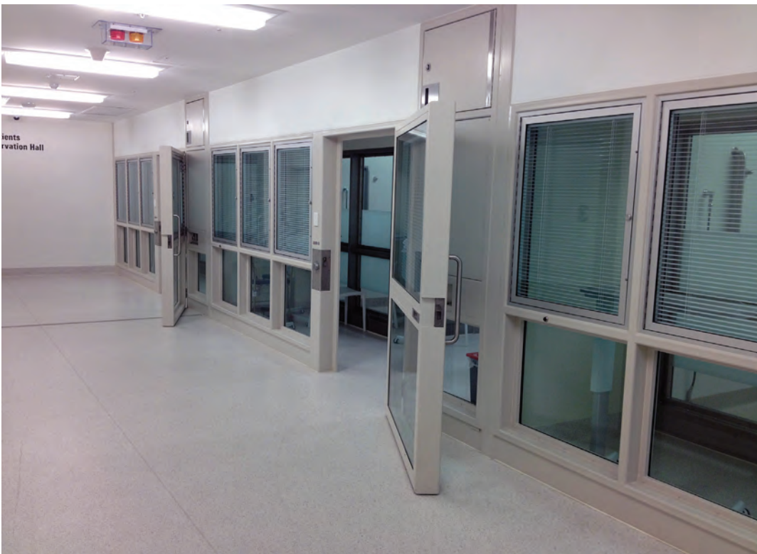
Figures 6 and 7: The new secure facility at Fiona Stanley Hospital
