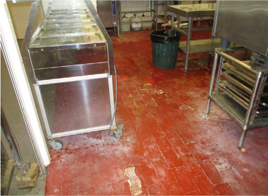
Figure 8: The damaged and dangerous kitchen floor
