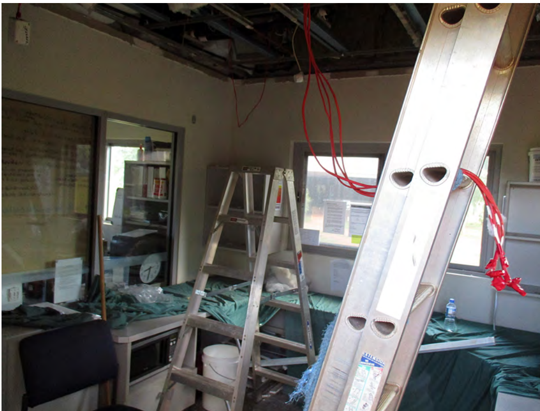
Figure 14: Unit 2 office ceiling destroyed by water
