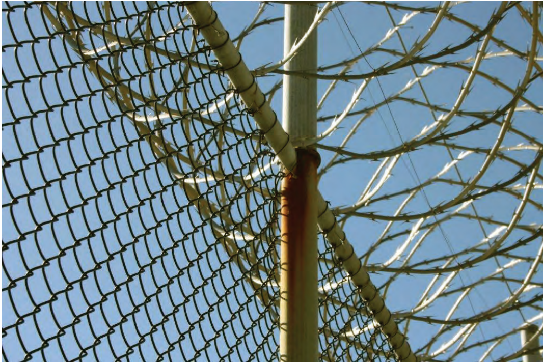
Photo 11: Rust erosion visible on perimeter fencing
