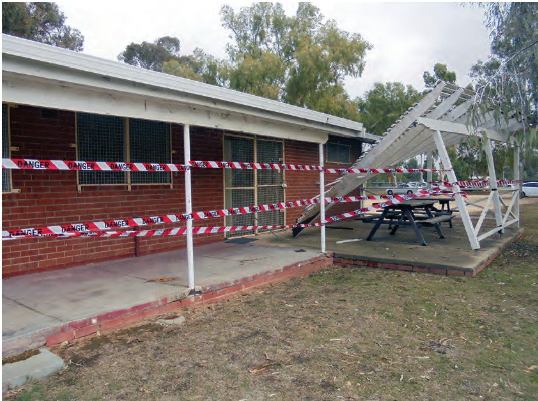
Photo 12: This disused building is a public safety hazard
