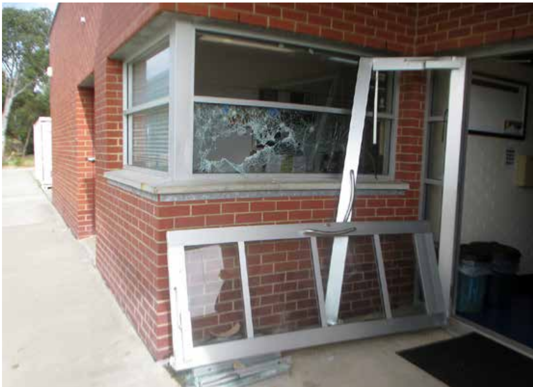
Photo 3: Damage caused during the May incidents
