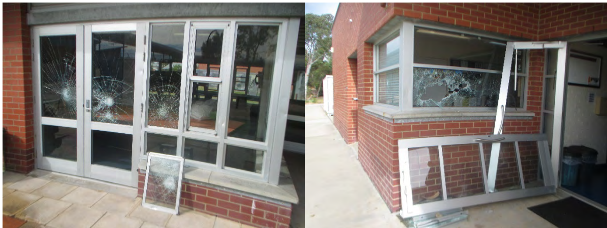
Photo 1 and 2: Damage caused during the May 2017 incidents
