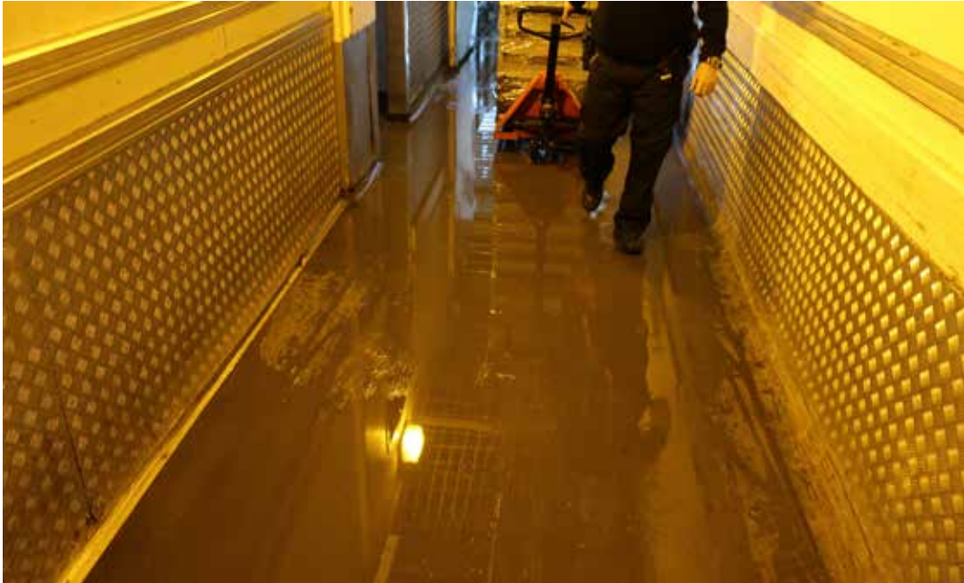
Photo 3: Water that has pooled in the kitchen
