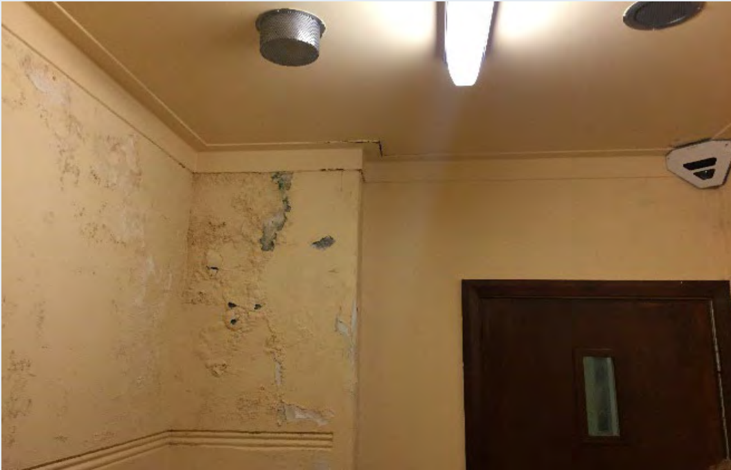
Photo 21. Supreme Court water damage
