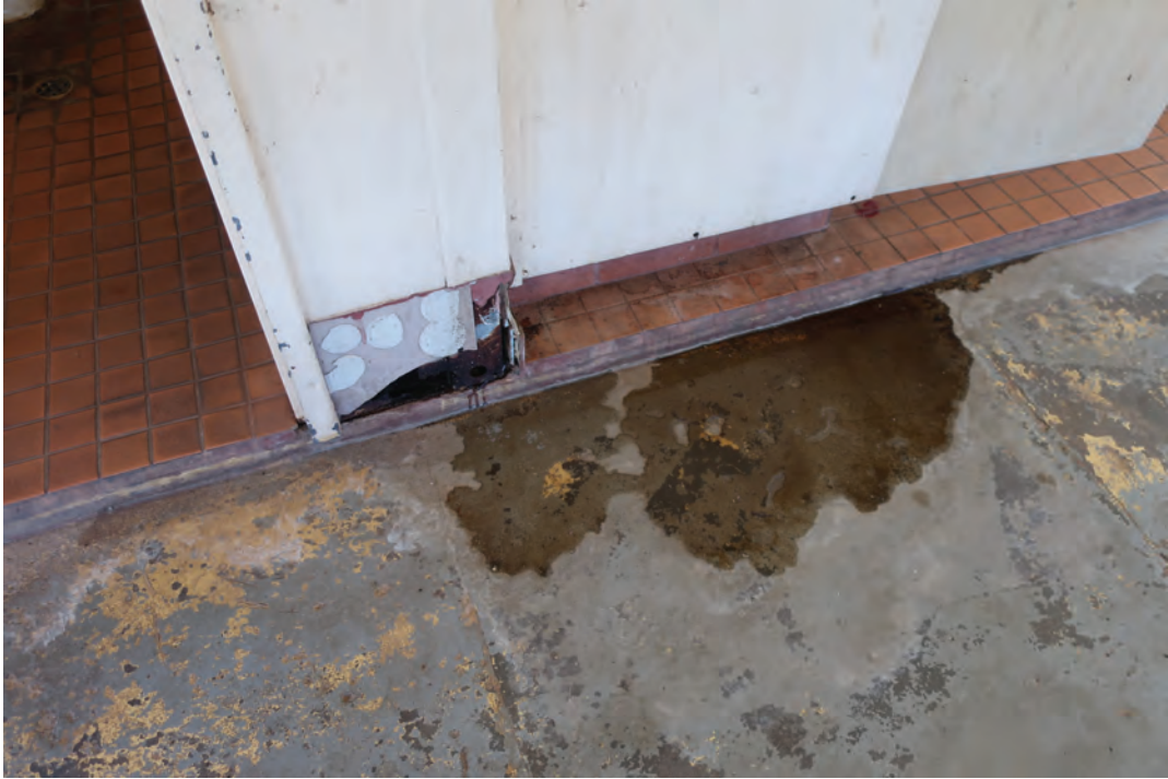
Photo 4. Mould and water damage continued to cause maintenance problems across the site.
