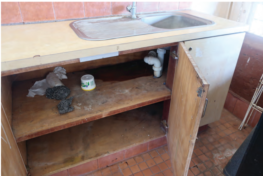
Photos 2 and 3. Mould and water damage continued to cause maintenance problems across the site.
