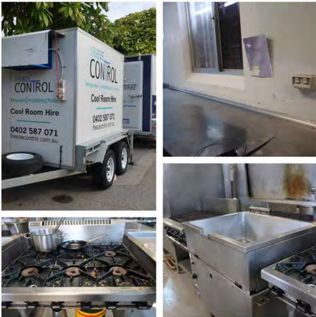
Photo 4: Additional cold storage, kitchen walls and equipment in poor condition
