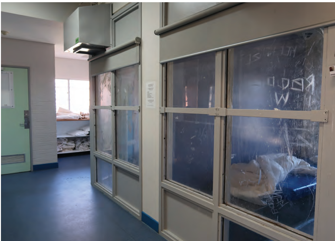
Photo 5: Observation cell windows were scratched and damaged.
