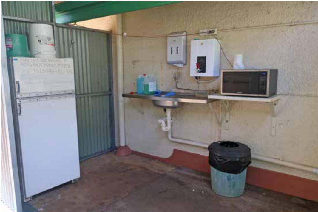
Photo 2: Outdoor kitchenette installed in Unit 2 and Unit 3
