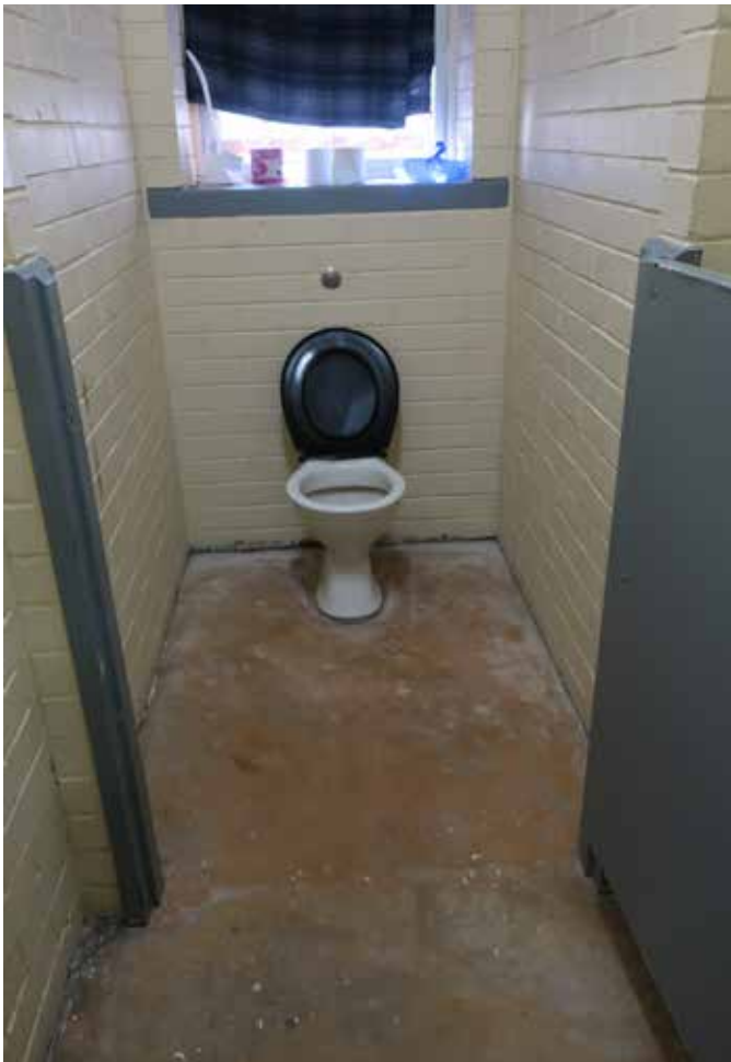
Photo 9: Flooring in bathroom of Unit 3
