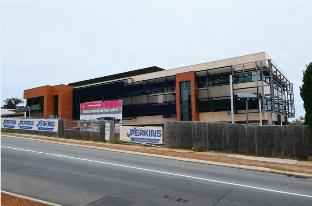
Photo 12: Armadale Courthouse and Police Complex: expected completion 2023
