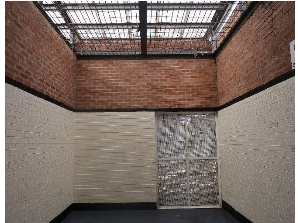
Figure 9: One of two D-wing yards from Unit 1 at Hakea Prison with no visibility of the sky.
