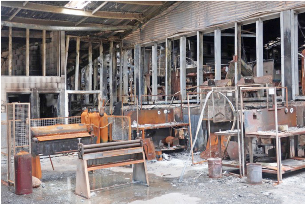
Photo 9: Significant damage was caused to Acacia's industries workshops during a disturbance in February 2022
