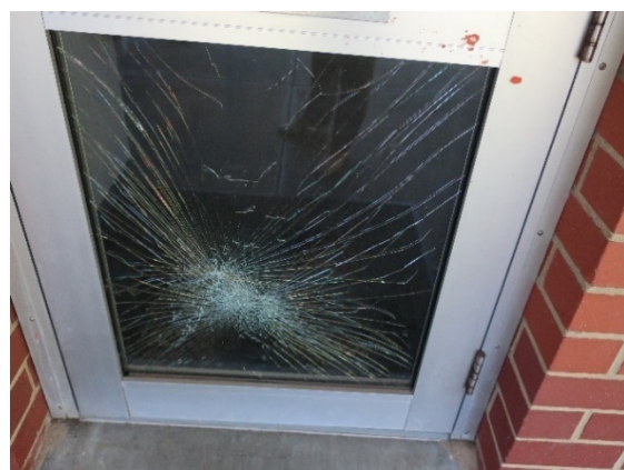
Photo 9 Broken glass needs urgent replacement
