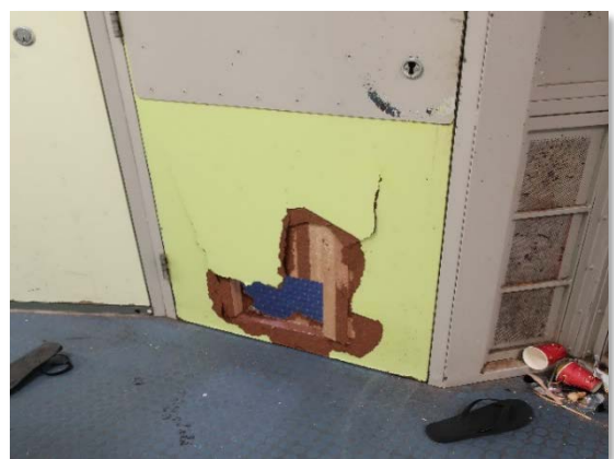
Photo 8 An out-of-order cell due to significant damage to the door with rubbish piled outside
