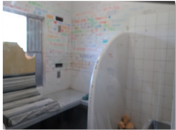
Photo 7 Extensive graffiti written over cell walls
