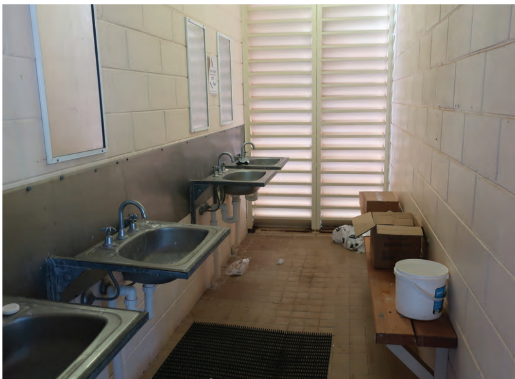
Photo 4. Minimum security ablutions were degraded
