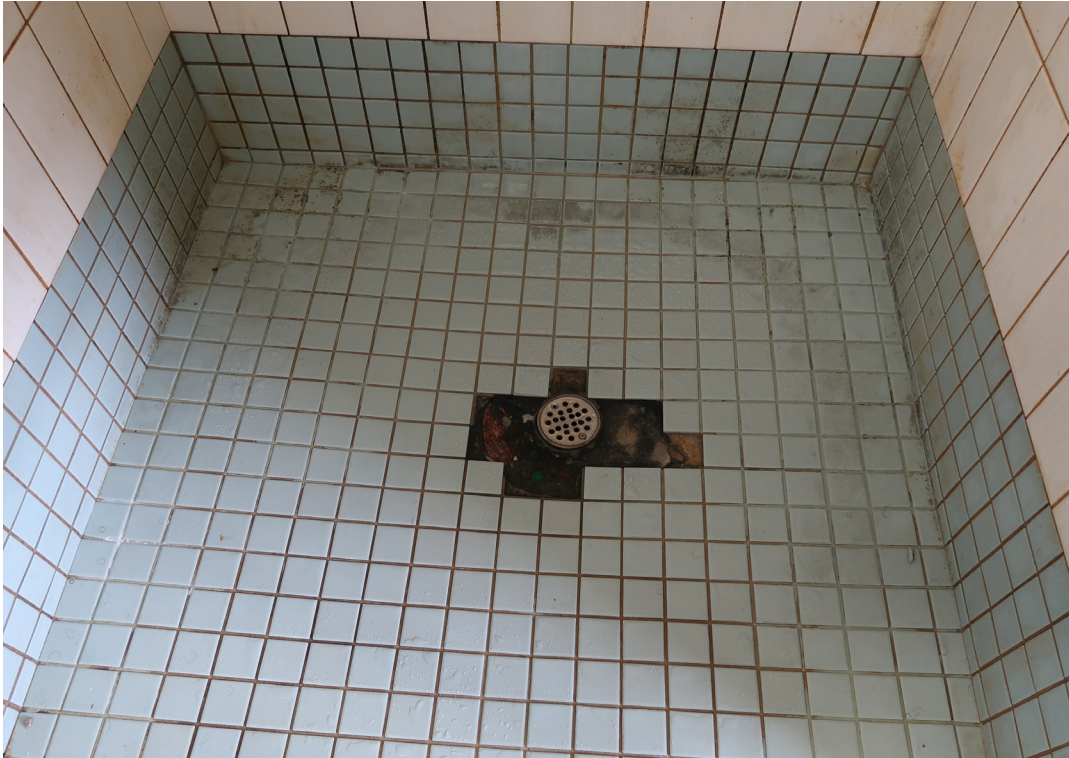
Photo 3: Grimy and damaged tiles in a communal shower.
